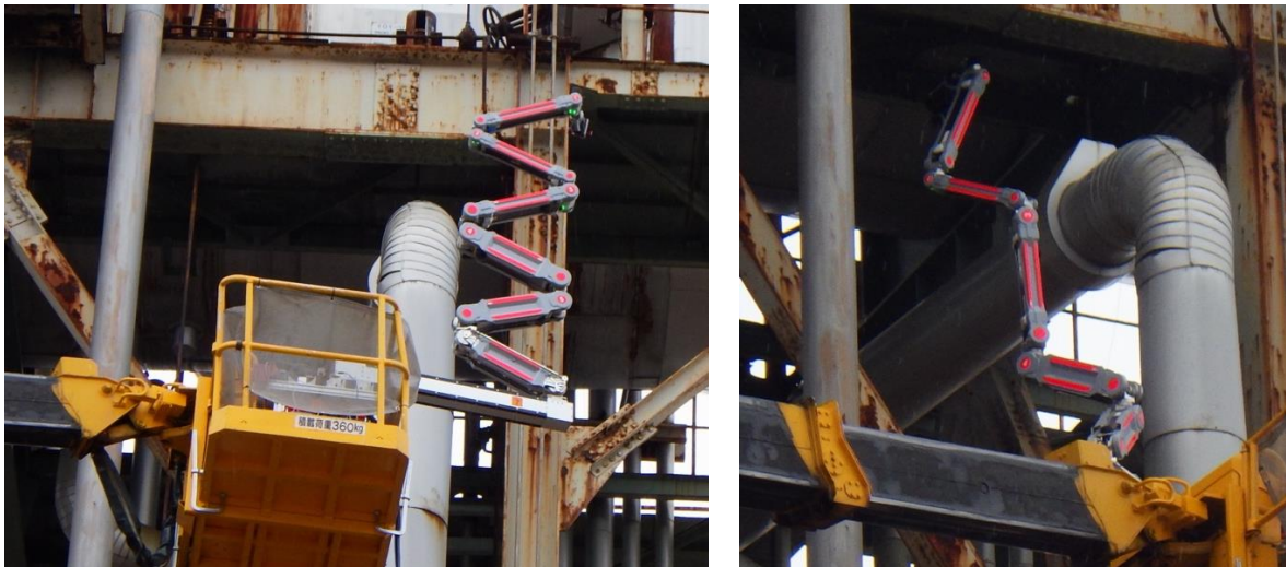
Float Arm during inspection mission at the Mitsui Chemical plant in Osaka
